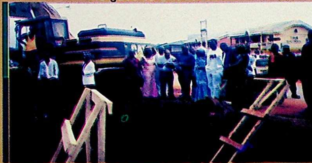
Governor Obi inspecting the foundations of the UNIZIK Pedestrian Crossing Awka, which some people claimed they did 50% of the job. The structure is now 85% completed
