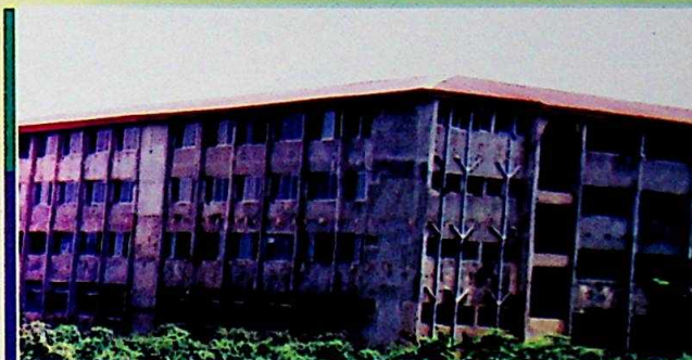
The office complex for Hon. members of the State House of Assembly under construction
