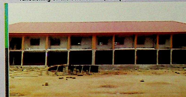
St. Charles College Onitsha, one of the schools being constructed by a corporate organization through Governor Obi's intervention
