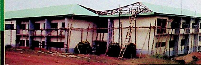
Agulu General Hospital: one of the 16 general hospitals Governor Obi is rehabilitating across the state; some others are the General Hospitals at Umuchu, Ukpok, Ossamala, Enugwu-Ukwu, Oraifite, Amanuke, Okija etc
