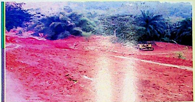
Work is on-going at Umuchiani Erosion Site. The Governor is working on many erosion sites in the State.
