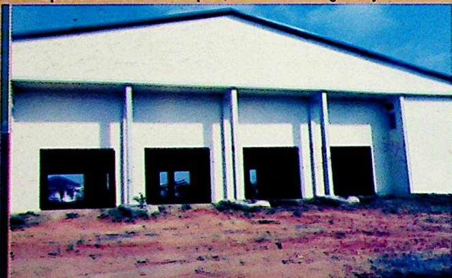
A new Fire Fighting Vehicle House completed for the State Emergency Management Agency (SEMA)
