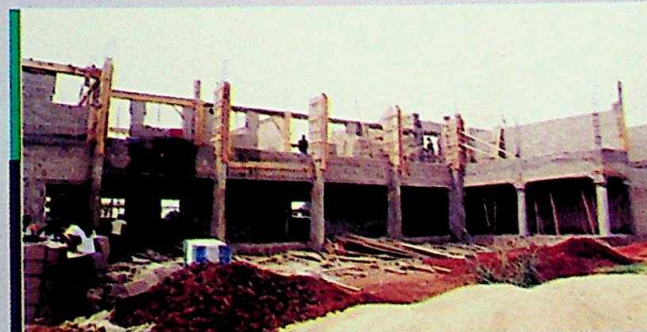
A modern classroom block under construction at Nwafor Orizu College of Education, Nsugbe. Due to inadequate classrooms space, students take lectures under trees
