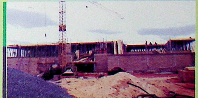
The Prof. Kenneth Dike Central Library under construction, the first library being built in the State since 1966
