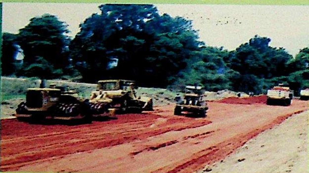
Work is going on aggressively on Umueze Anam-Mmiata Road, the first road construction undertaken by any Government in Anambra West Local Government Area since the State was created
